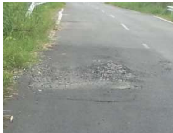
b. Distortion on road pavement
