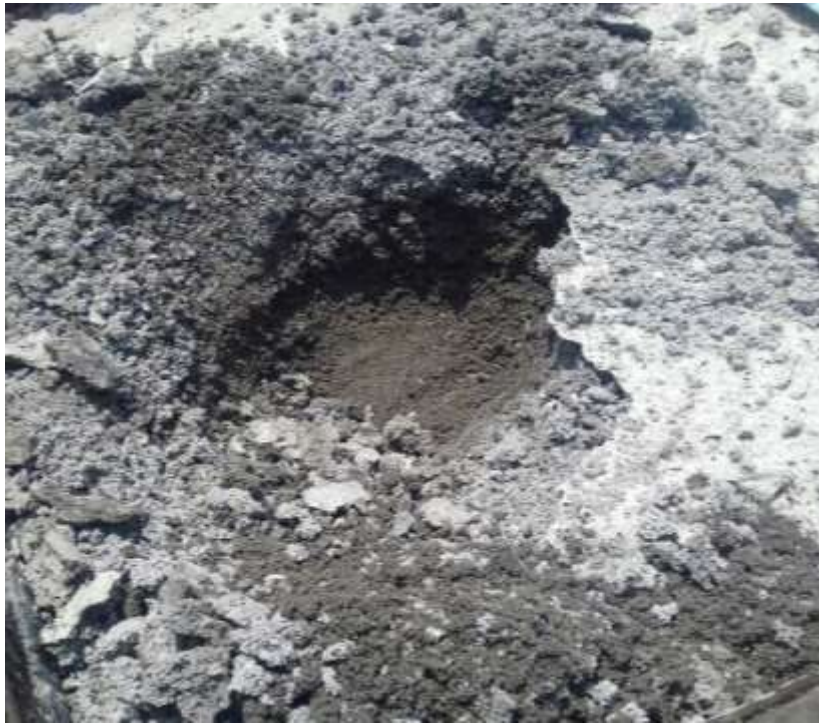
Figure 5.6: Foamed concrete become fragile with w/c more than 0.35
