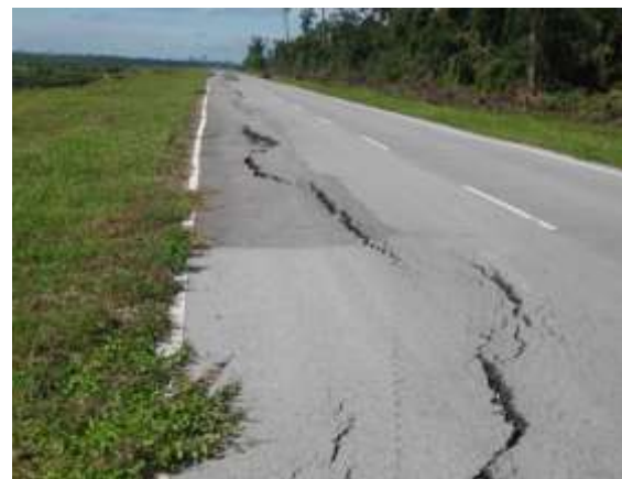
a. Cracking on road pavement
