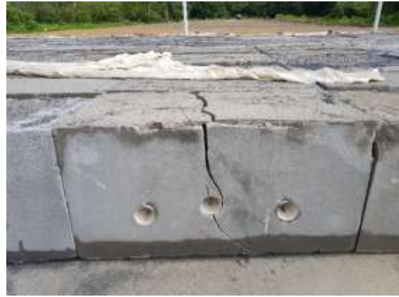
(b) Crack on the block is not allowed
