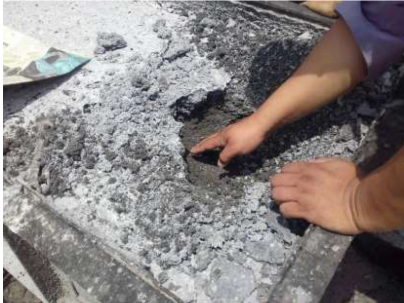
Figure 6.4: Foamed concrete segregation and fragility
