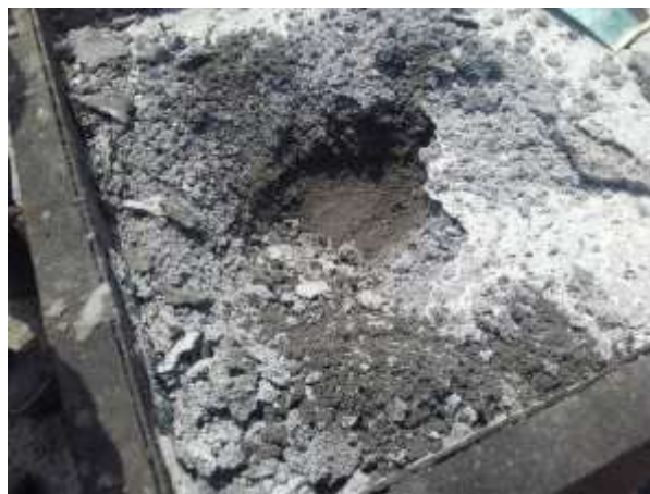
Figure 4.3: Foamed concrete with segregation
