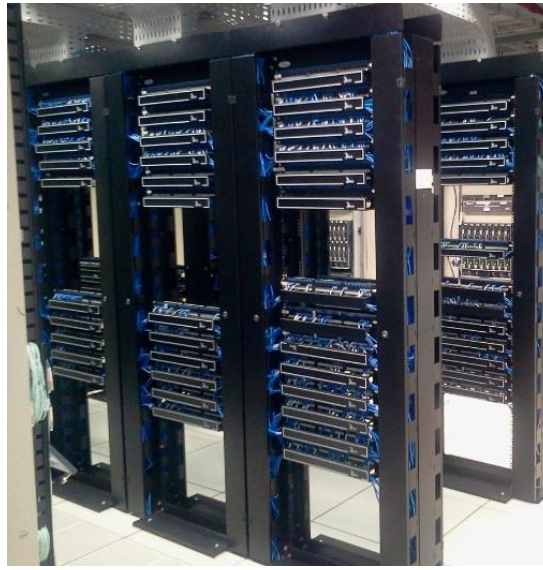
Figure 32: Picture of Several Web Servers on server racks
