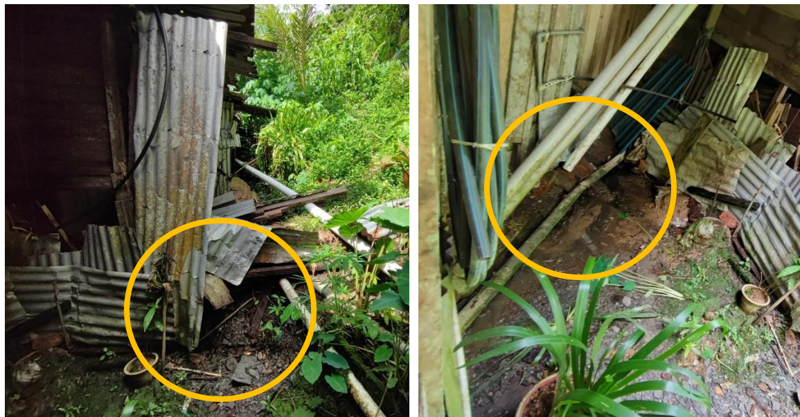
Figure 4.9: The landslides happened in one of the longhouses in Nanga Entawau
