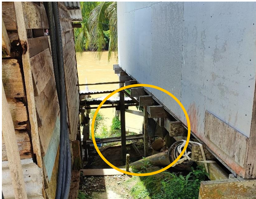
Figure 4.8: The picture on the land sliding situation on the longhouses in Nanga Entawau nearby the Baleh River
