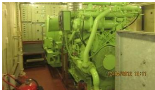
Figure 2.5.3: Machinery Installation (Hasan, 2019)
