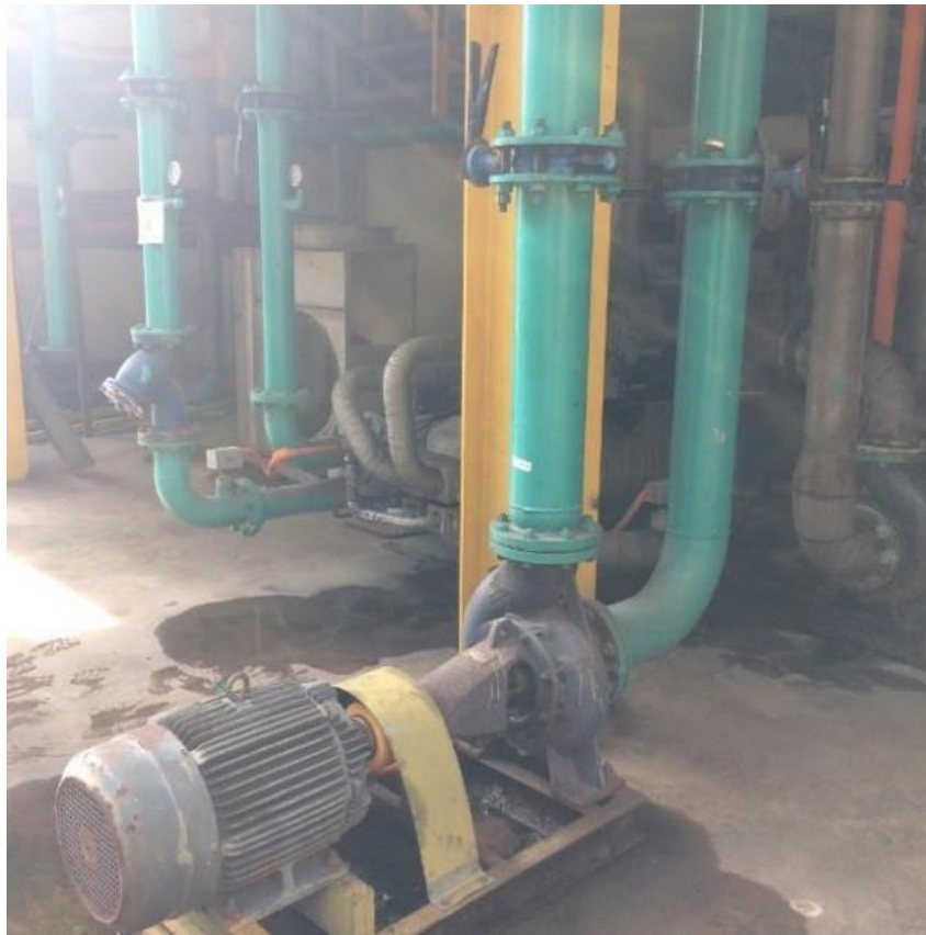
Figure 4.4: Targeted Pump at Plant A
