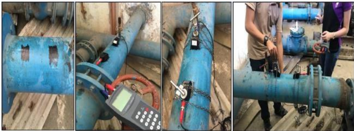
Figure 3.2: Installation of flow meter to calculate the flow rate of the pump
