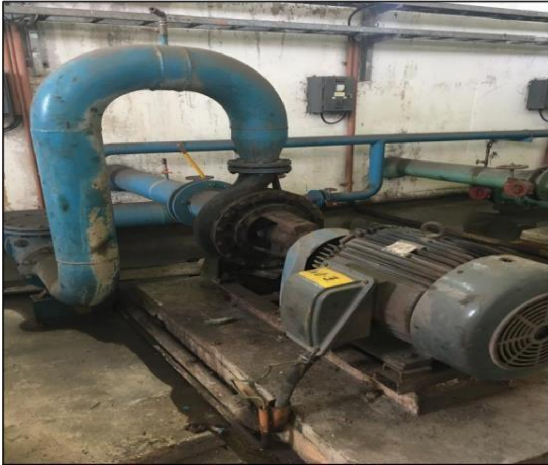
Figure 4.11: Targeted Pump at Plant B
