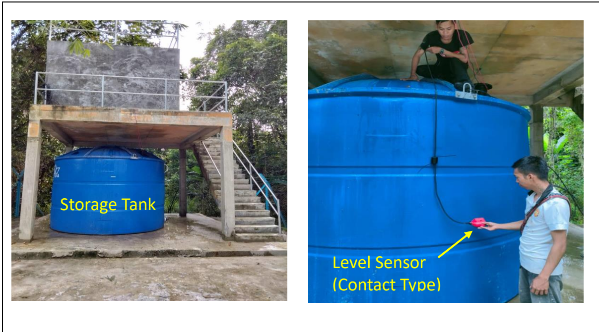
Figure 3.3 (b): Storage Tank and Level Sensor Set Up
