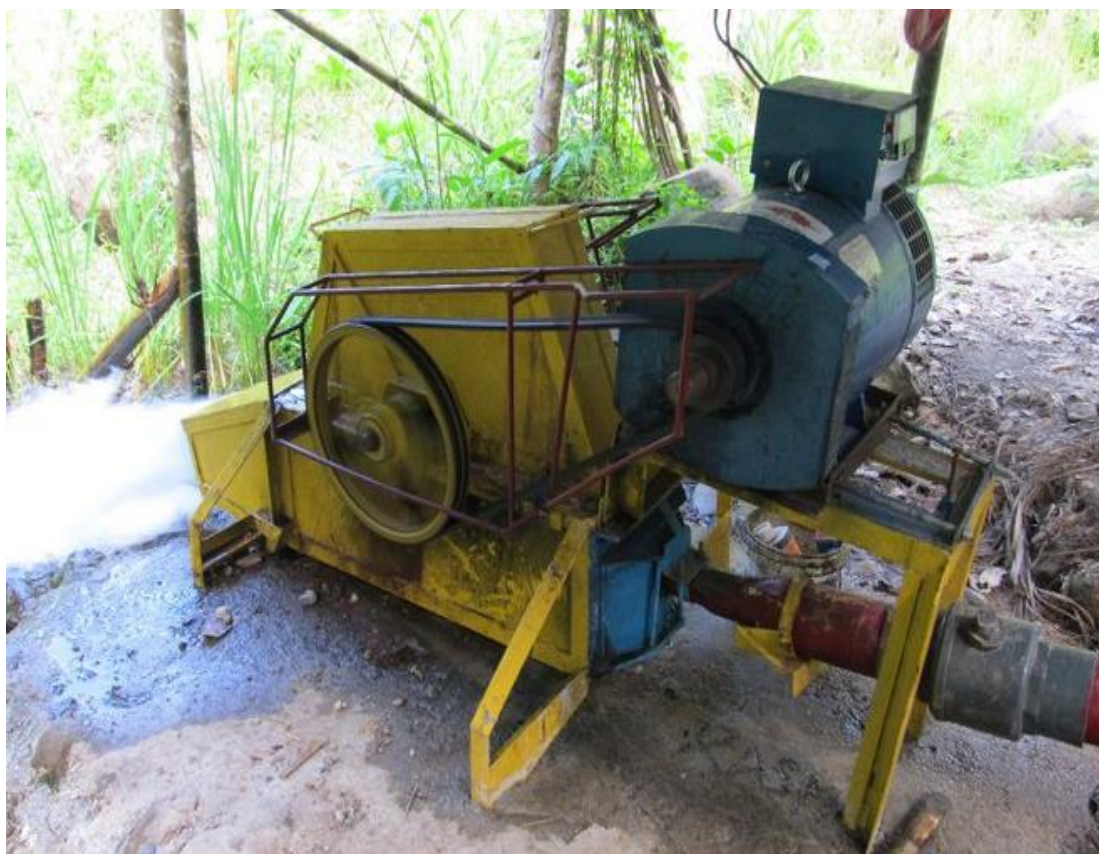
Figure 2.1: A 10 kW MHP at a rural village in Sarawak (Bombastic Borneo, 2011).
