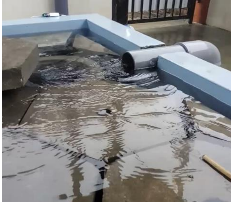
Figure 4.5: Overflowing due to 22 February 2020 Storm Event
