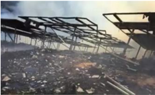
(c) Village-Level Photovoltaic Power Station
