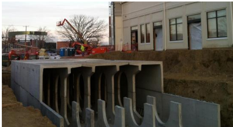
Figure 2.11: DoubleTrap used in Storrs Center, Village Steet, Mansfield, CT (StormTrap, 2018)
