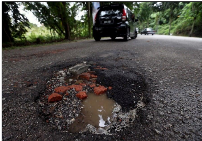
Figure 2. 1: One of the potholes in Malaysia
