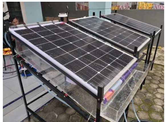
Fig. 4. Application of water cooling systems
