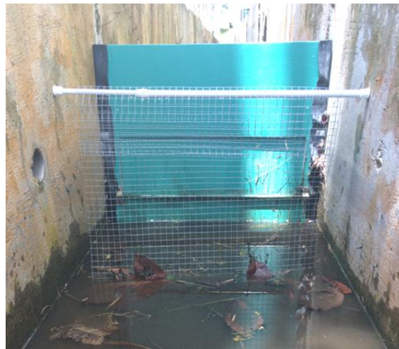
Figure 4.17: A trash trap with one end fixed was installed
