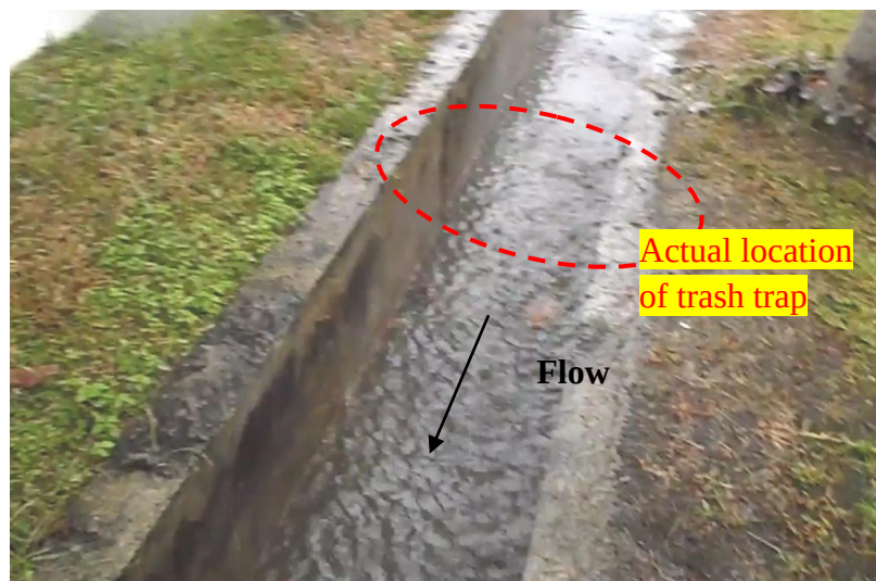
Figure 4.21: Trash trap was flushed off and fully submerged in water
