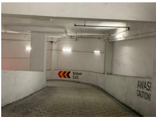
Going down through a dangerous slope 1
