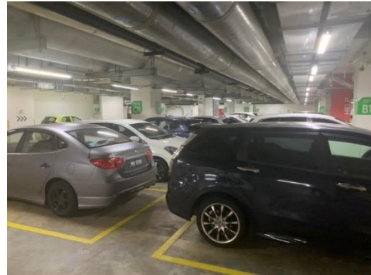
Parking sensor is not functioning (no green lights)
