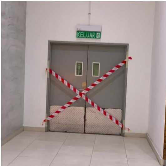
Closed exit doors
