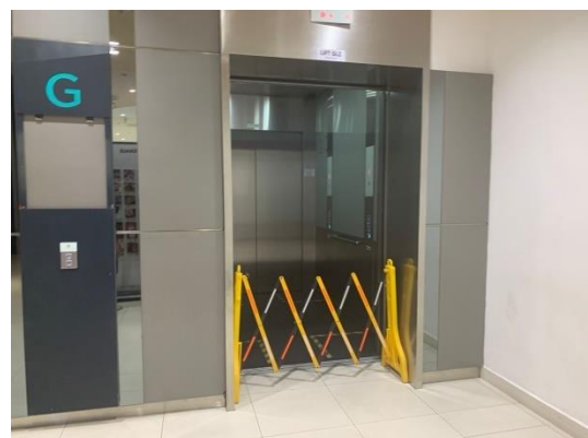
Malfunction lift in Level G
