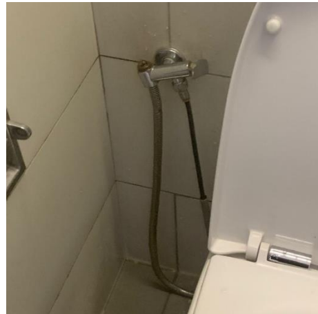
Broken water hose
