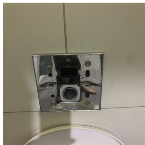
Broken toilet pump
