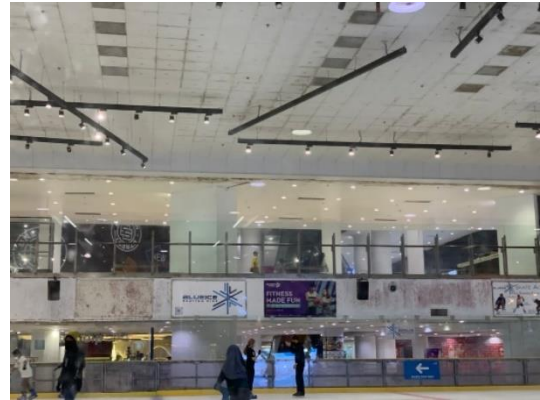
Mould/mildew on the ceiling of ice rink
